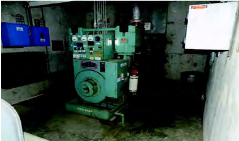
235-F Diesel Generator
