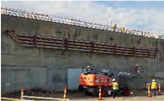
Cooling Water Lines-Before
