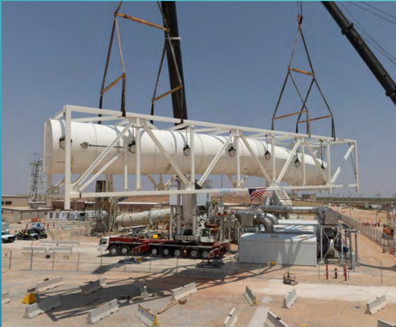
Installation of the ductwork bridge that will connect the existing underground ventilation system to the SSCVS when it comes online.
