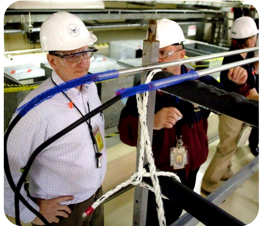
Replacement of containment electrical penetration assemblies at the Fort Calhoun nuclear power plant
