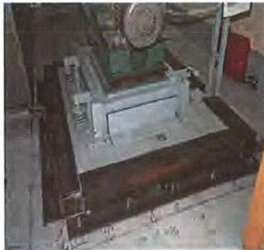
Figure 4. Glovebox Exhaust Fan and Concrete Base Pad with Bracing shown on the Perimeter of the Fan Pad
