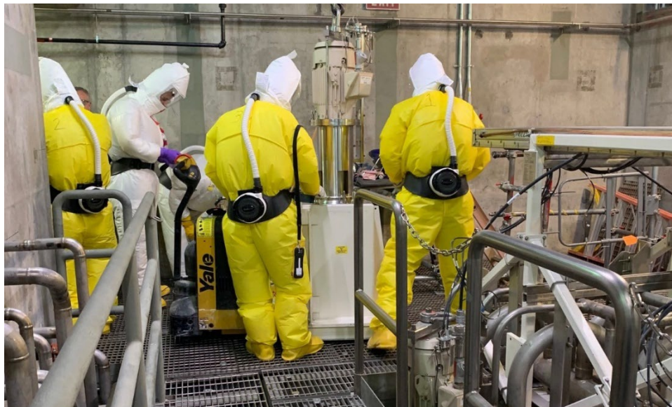
Facility's Personnel Demonstrate Replacing a Contactor Prior to Start-up
