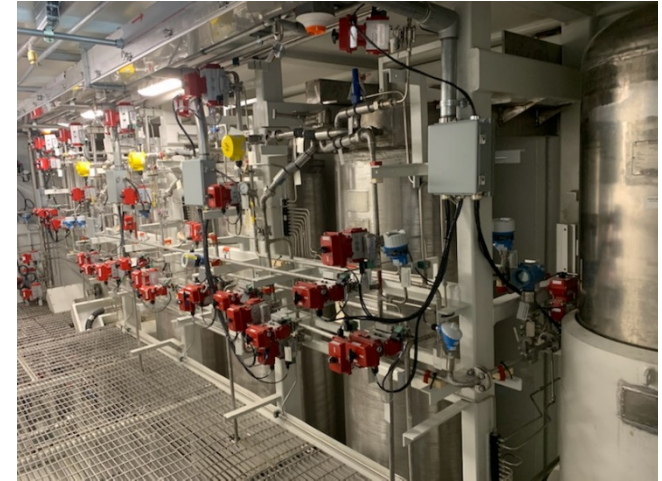
Tank Side Cesium Removal System Process Enclosure
