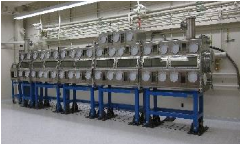
LLNL Plutonium Facility Recovery Glovebox Line
