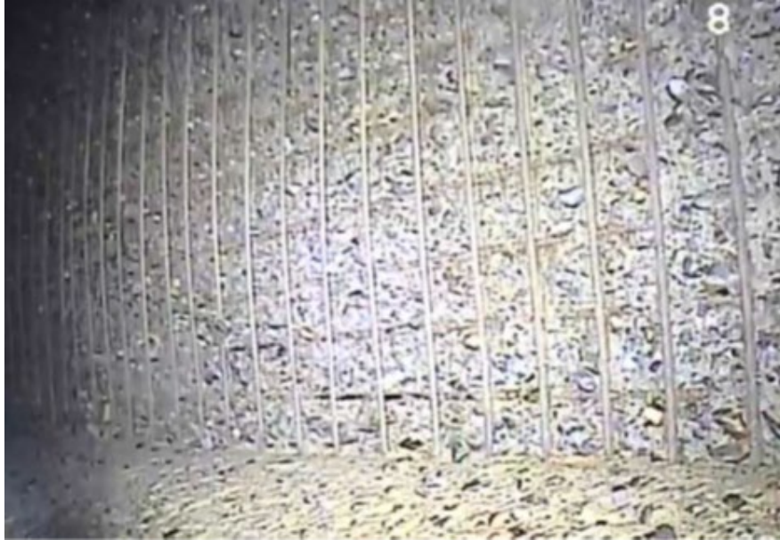
HCAEX Tunnel Wall Showing Concrete Loss and Exposed Rebar
