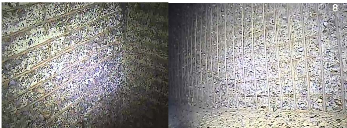
Figure 2. Stills from 2014 crawler inspection video showing two layers of exposed rebar. Degraded concrete debris can be seen accumulated at the bottom of the wall (right).
