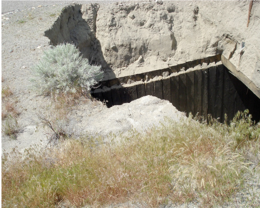
Partial Collapse of PUREX Tunnel #1
