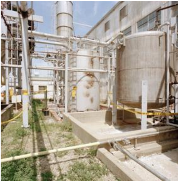
Chemical storage tanks at Fernald (1994)
