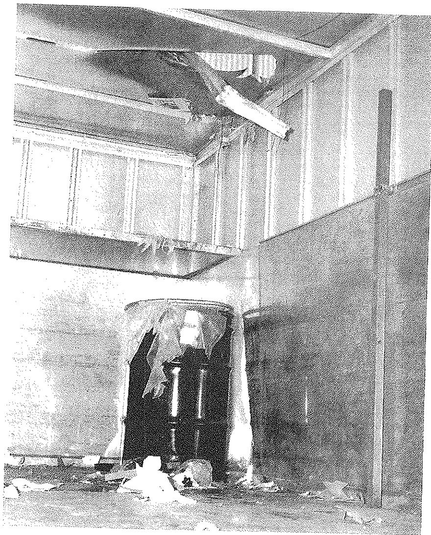
Fig. 1 Damage inside a truck at Argonne National Laboratory-East caused by the explosion of a 55-gal drum containing mixed radioactive waste. Published with permission of authors and the U.S. Department of Energy.
