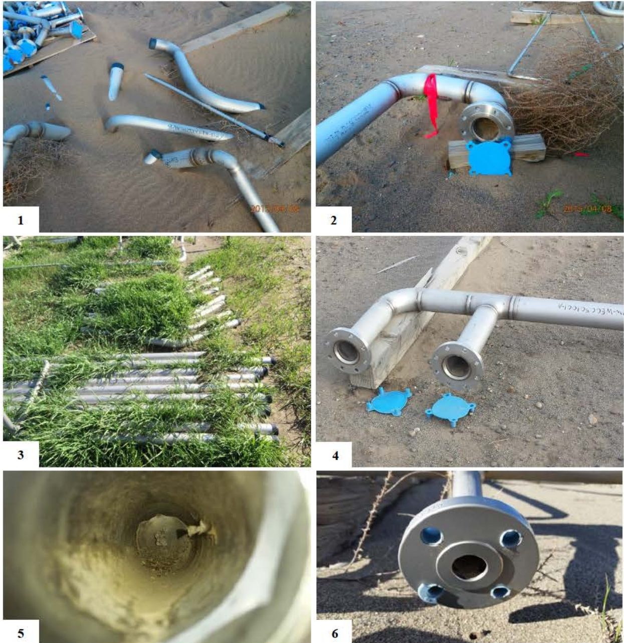
Figures A-1 to A-6. Staff review team photographs illustrating deficient storage conditions at the Material Handling Facility (MHF) Laydown Yard. Figure A-1 shows pipes buried in the sand. Figures A-2, A-4, and A-6 show missing pipe caps on pipe modules and a layer of sand built up inside. Figure A-3 shows excessive vegetation surrounding pipe modules. Figure A-5 appears to show part of an insect nest inside a structure, system, or component (SSC).
