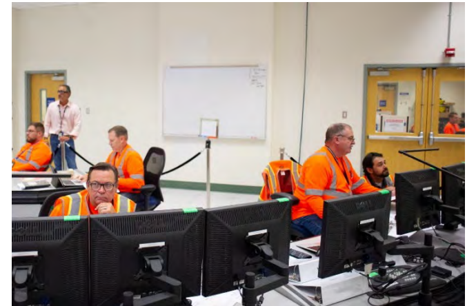
LAW Facility Control Room
