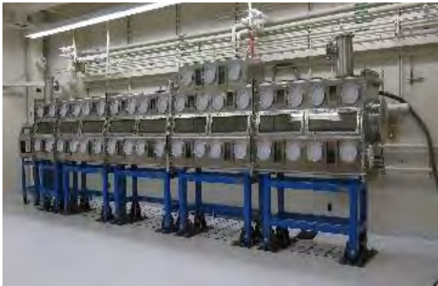
Recovery Glovebox Line
