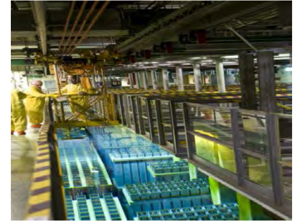
L-Area Spent Fuel Basin
