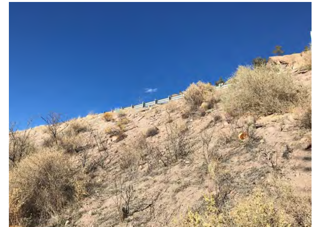
Cliff Alongside Transportation Route in Los Alamos
