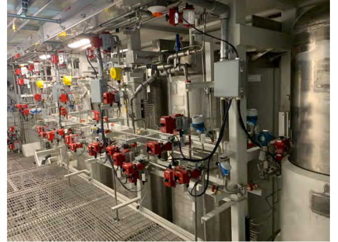
Tank Side Cesium Removal System Process Enclosure
